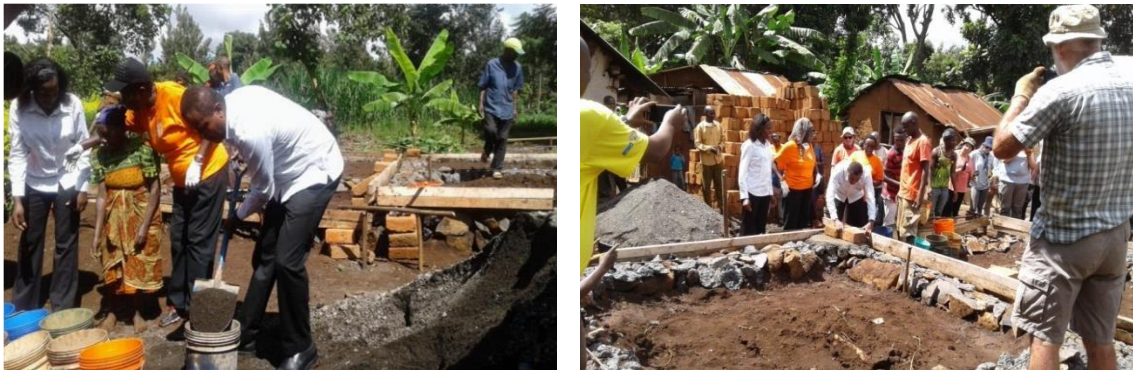
Figure 9. In April 2018, the Moshi District Commissioner Hon. Kippi Warioba (in white shirt) participated in the gravel mixing and laying the first brick on the 100th House supported by the Vine Trust of Scotland
